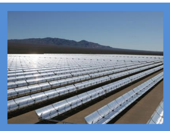
Nevada Solar One
